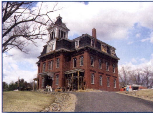
The Tri-County Community Action Program recently celebrated its successful renovation and adaptive use of the Ashland School (shown here with construction nearing completion).
